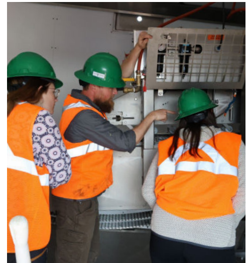
Safety Manager Jacob Mannix gives Lizzy and Sonja a tour of the NSSP plant facilities in Nome.
